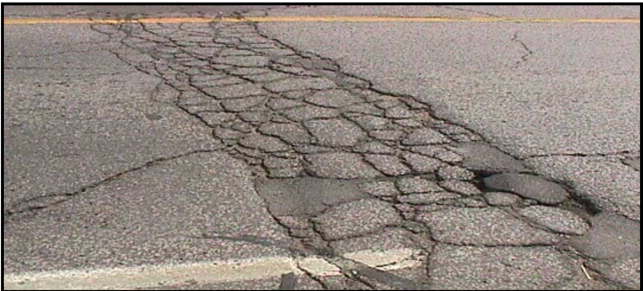
Figure 6: Utility trenching permanently damages roads
