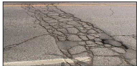
UTILITY TRENCHING DAMAGES ROADS
