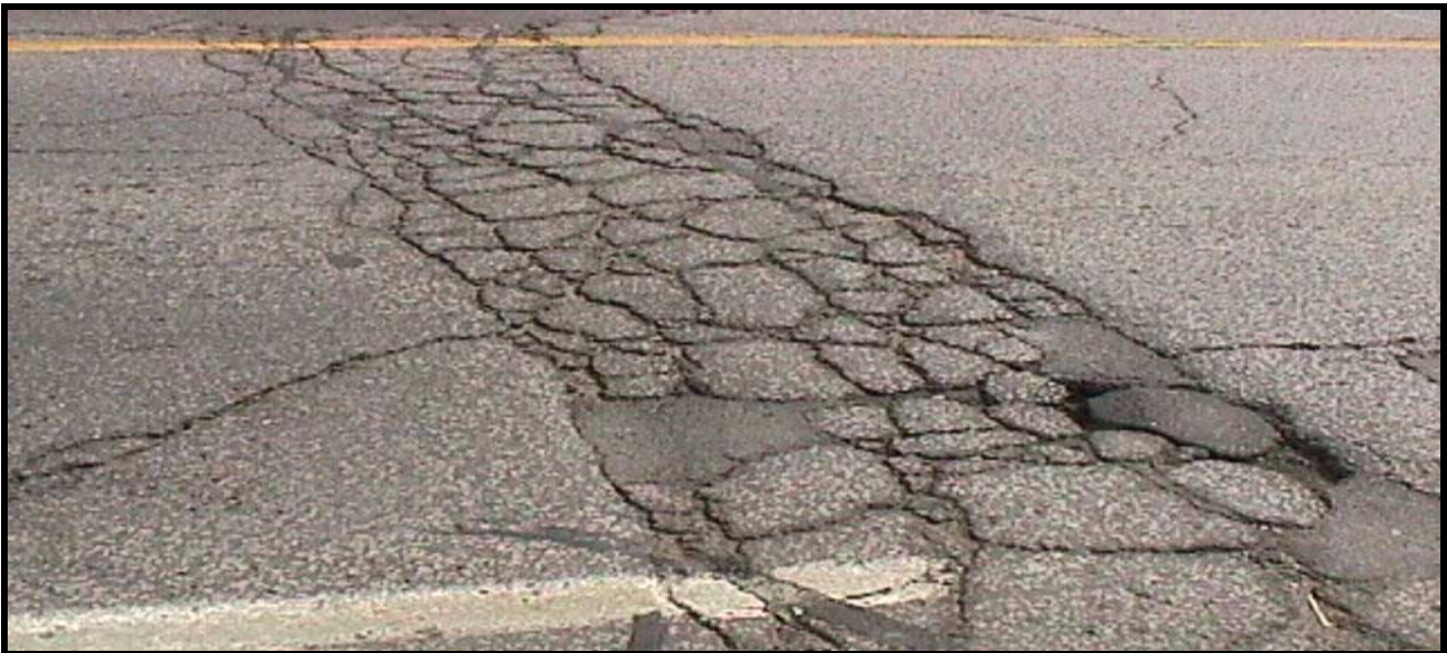
Figure 6: Utility trenching permanently damages roads
