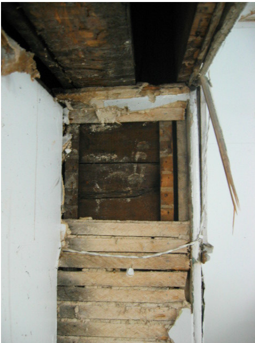
Fig.9 Interior view of the mansard roof, showing remnants of lath and plaster, with wood corner bead, and 3"x6" framing member above.
