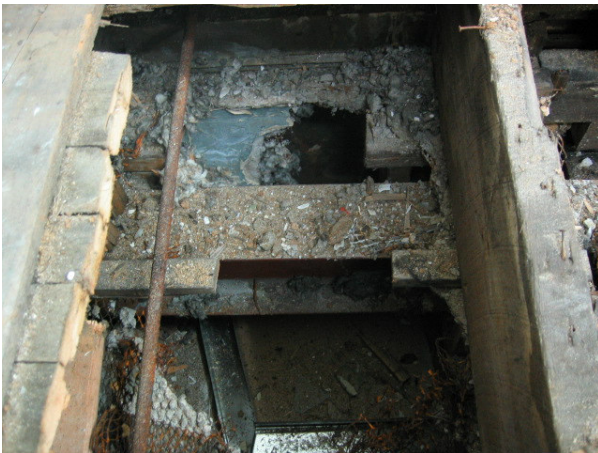
Fig.4. The original hardwood floor is visible on the left, above the 2x10 wood joists @ 24"o.c. Immediately below is one of the series of east-west 8" deep steel beams, and below these is a welded bracket and a 14" deep north-south steel beam.
