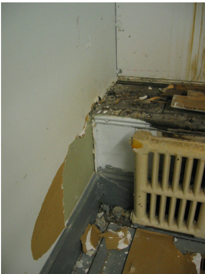
Fig.7 details showing intersection between bearing wall (left) and middle dormer (right). Original lath and plaster finish is visible behind later drywall. Baseboard and window sill are original.
